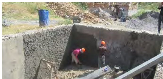
Rehabilitation of water infrastructure in Dahana, Kulyab. Source: 2 Quarter 2018 Report by PMO SUEKMK
